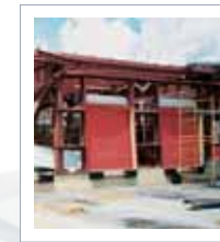
After Hurricane Andrew in 1992 our Model 651 door was the only item left on the building.
